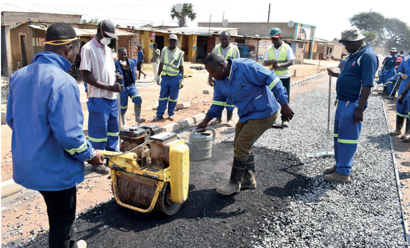
Kenyan trainer Johab Oteno Osika (with a watering can) showing contractors how to compact the cape seal during practical training session on the Lubombo Road.
